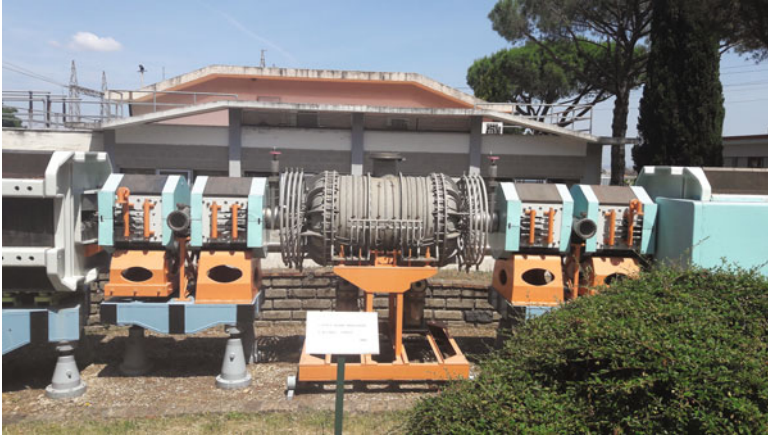
Fig. 3.7 Example of a FODO cell hosted at the LNF site: a magnetic dipole is followed by a pair of quadrupoles with alternated polarity, and by a RF cavity
